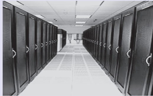
Fig 2: Cabinet aisle in a data center
